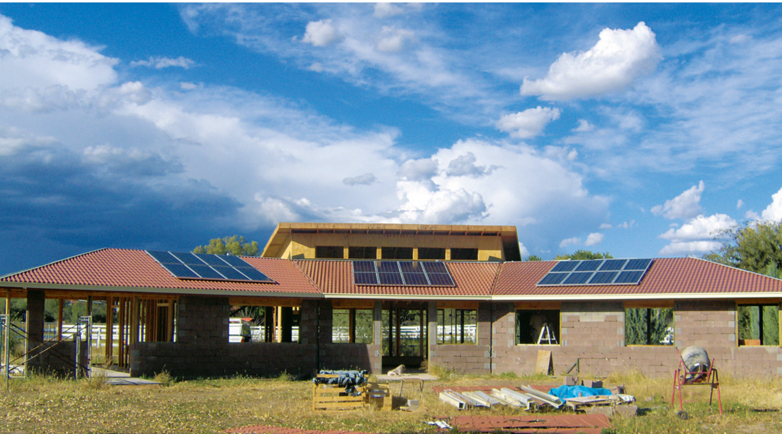
Three sets of photovoltaic panels will provide most of the electrical requirements for this home under construction.
